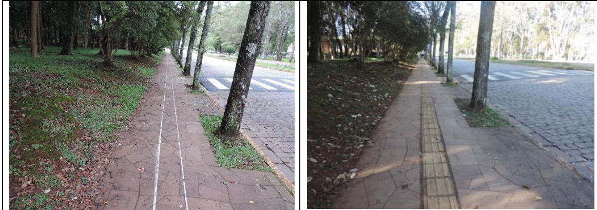
Figure 5. Sidewalk before modifications and in the stage of the project implementation. Source: Authors, 2015.
