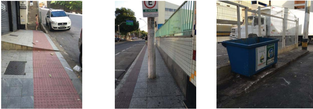
Figure 6: Incorrect execution of citizen sidewalk pattern and location of inadequate public spaces fixtures.
