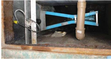
Figure 4. Parshall flume and ultrasonic level sensor
