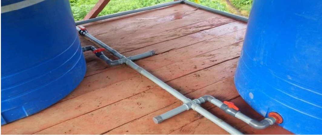
Figure 4. Interconnection of the water storage tanks
